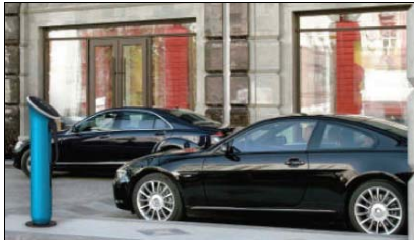
Figure 4 Commercial vehicle charging station
